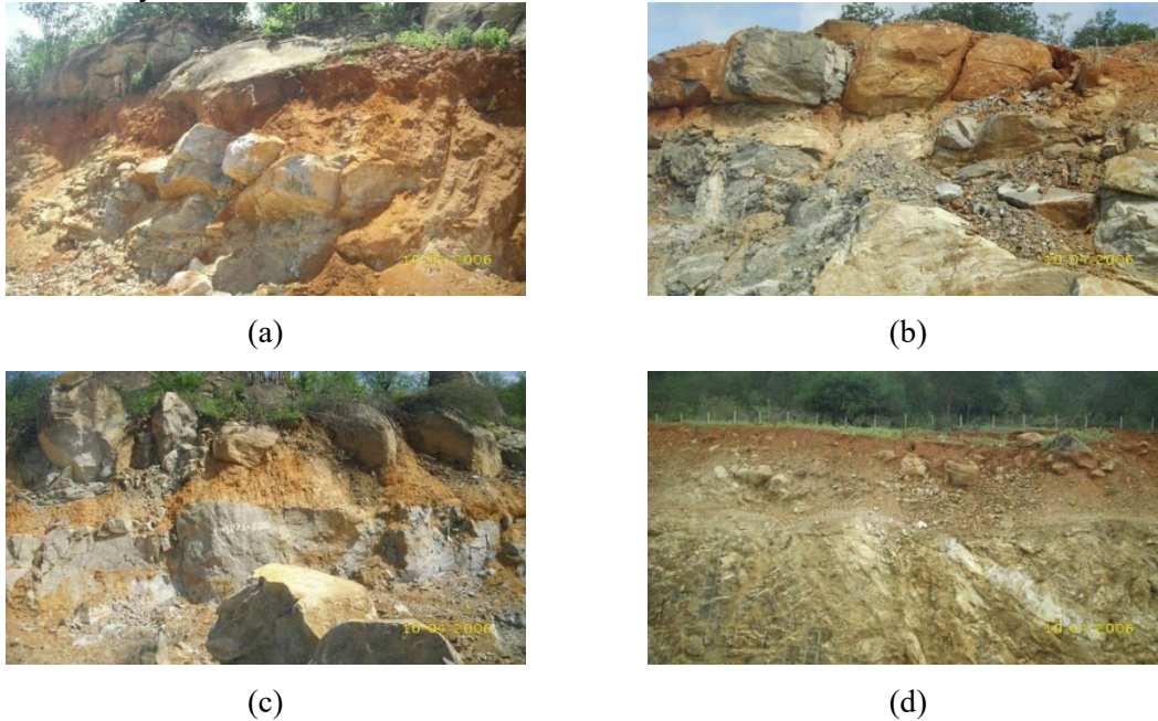
Figure 6. Presence of rocks in the crest of the excavation slopes: (a) ES 1264+040 - Cut 14; (b) ES 1268 + 640 - Cut 21; (c) ES 1271+880 - Cut 25; (d) ES 1275+540 - Cut 36
