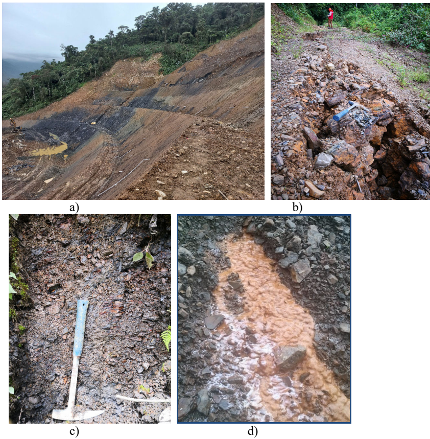
Figure 7. a) Cut of slope, grey color weathered rock, brown color residual soil. b) Cracks in slope and weathered rock. c) Residual soil. d) Oxidations and efflorescences of salts of shales and Slates.
