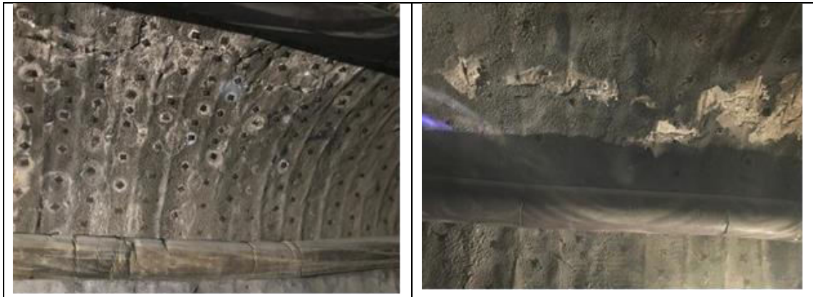
Figure 2. Some views from the cracks occurred after ring closure.
