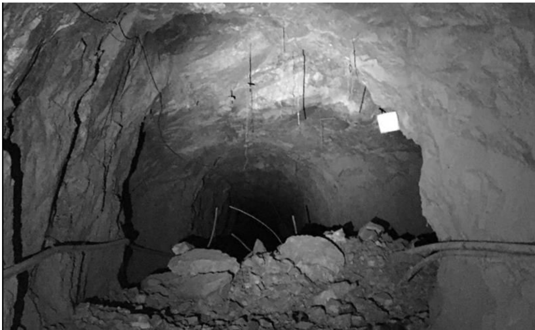
Figure 7. Stress relaxation in a jointed rock mass causing gravity failure of rock blocks from the back of the intersection of drifts (courtesy FF GeoMechanics, 2021).
