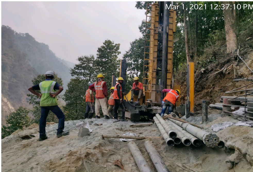
Photo- 3- Micro-pile installation work at top of slide zone for slope protection
