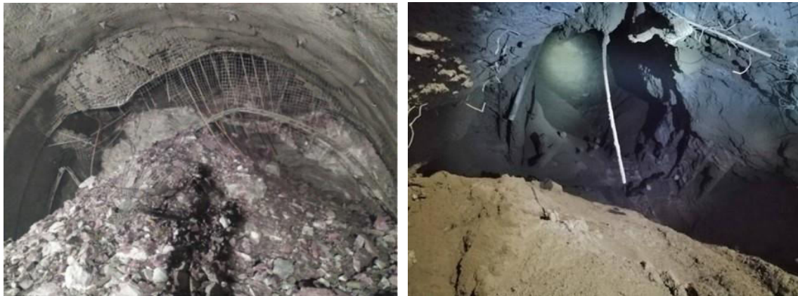
Figure 5. Loss of stability at the occurrence of cavern in the roof of the right tube of tunnel Ivan
