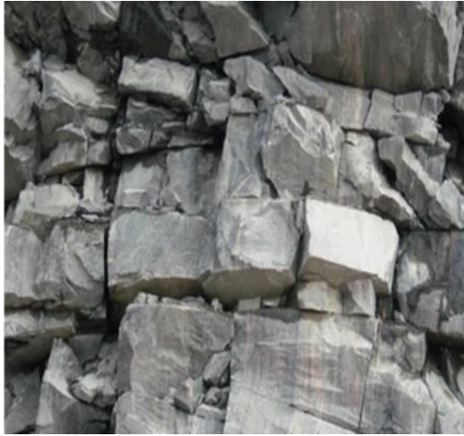
Figure 6. Cut slope in the discharge channel of the Tocoma dam in Venezuela.
