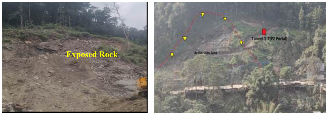
Photo- 1- View of Active slide zone and weathered, sheared and jointed rock mass phyllite, chlorotic schist are exposed at road cutting location on the way to T7-P2 Portal
